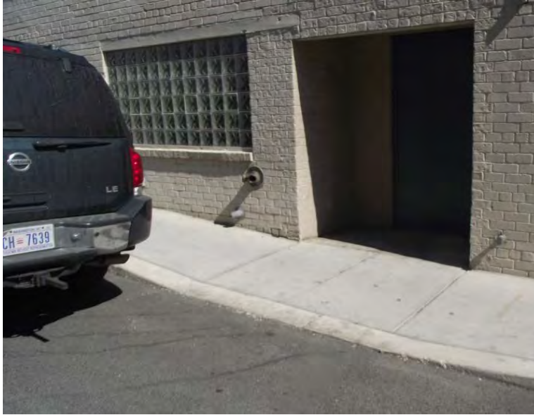
Figure 12 – Non-Standard Pedestrian Ramp at School Entrance
