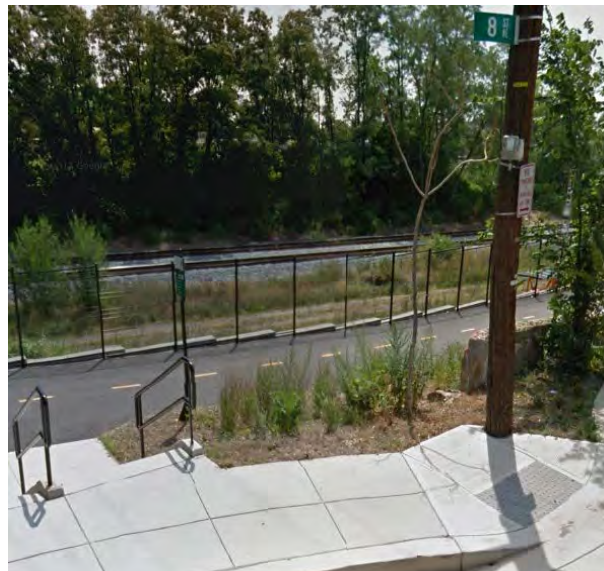
Figure 16 – Improper Pedestrian Ramp to MB Trail
