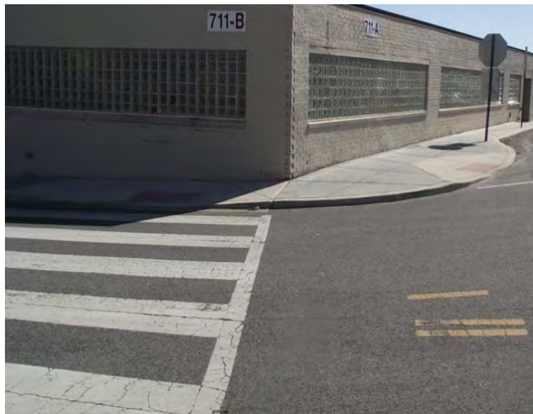
Figure 13 – Narrow Sidewalks at Pedestrian Ramp
