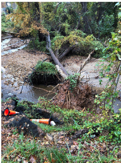
View of sidewalk at street level (Upper left image). View from street level down to forested area below (Upper right image). View of fallen tree and root structure (Lower left image).
