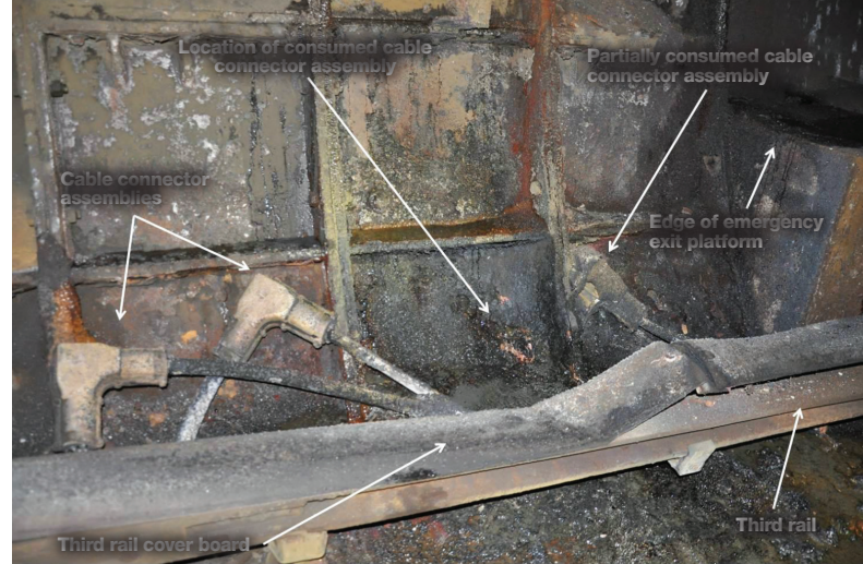
Fire-damaged cables and cable connector assemblies
